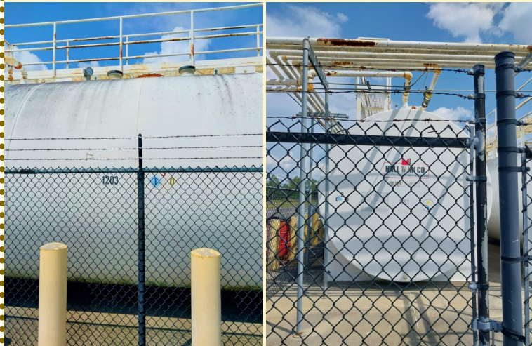
Before Photos: The fuel farm has rusty, faded areas of paint.
