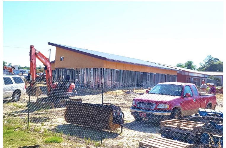
HeadStart/Early HeadStart Project is moving fast! Roof is on, power is being ran to the building, and the metal for interior walls can be seen.
