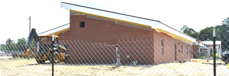
The City/County/action pact joint project for HeadStart/Early Head-Start new classrooms and kitchen addition is nearing completion.
