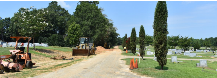
The Douglas Cemetery drainage and road improvement project has begun. Plans are to improve drainage, pave the dirt roads in the new section, and resurface some of the existing roads.
