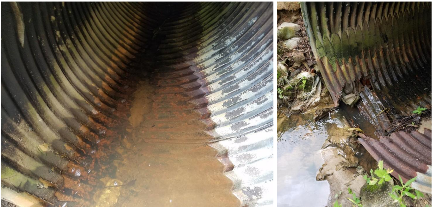
Failed Storm Drain Pipe Under E. Gordon Street
