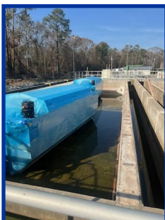
New Disc Filters at the Wastewater Treatment Facility.
