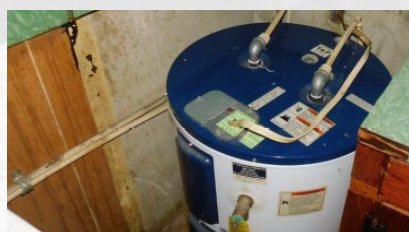
Replace old water heater & possibly relocate out of kitchen.
